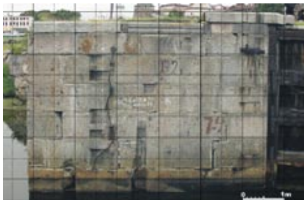
The northern entrance wall showing the various alterations and the crack, right, in the structure.
