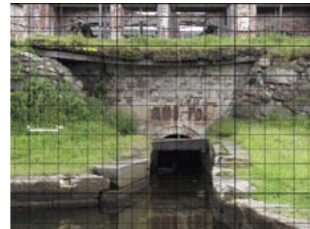
The dangerous section of road by the hydro-electric station outlet.
