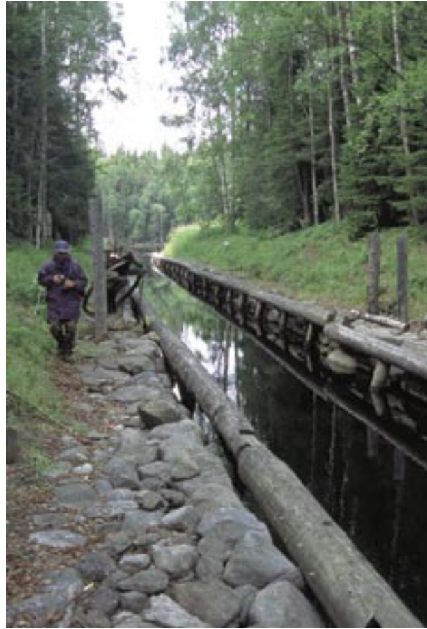
Canal K8 has been rebuilt, though the swing bridge crossing it still requires restoration.
