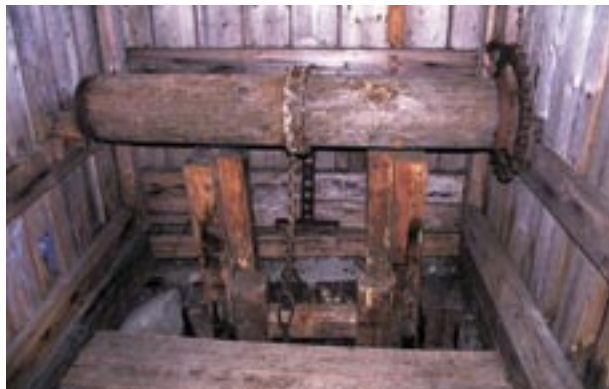
The mechanism of sluice 2.
